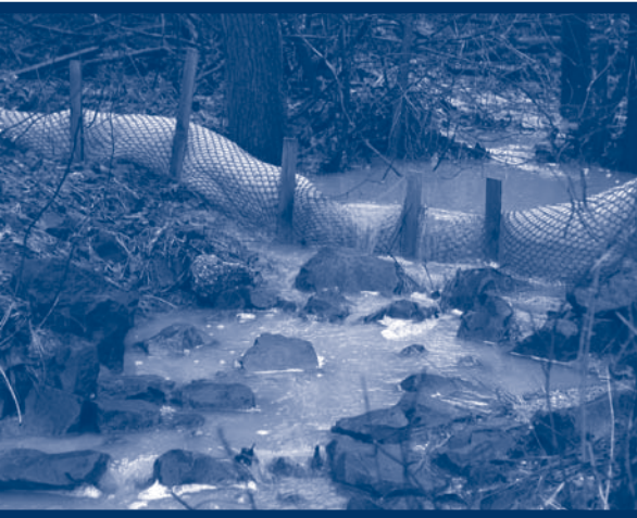
Filtration Tubes in a Channel
