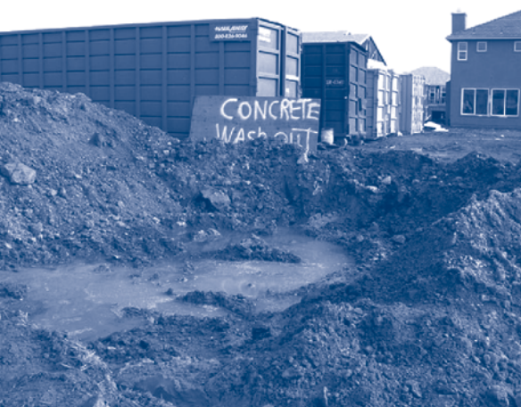
Example of Non-Compliant Washout Area
